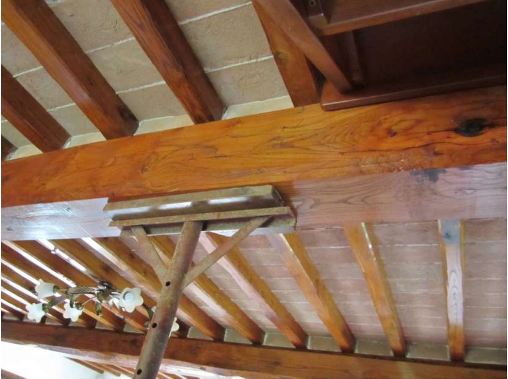
Support and crack
