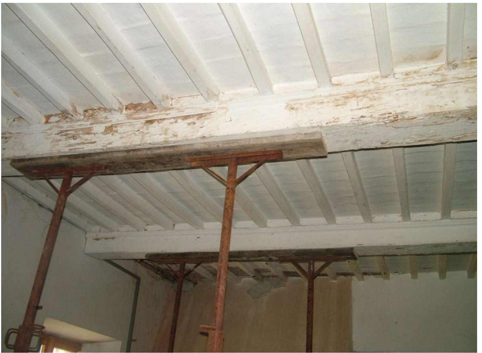
Detail of the supports
