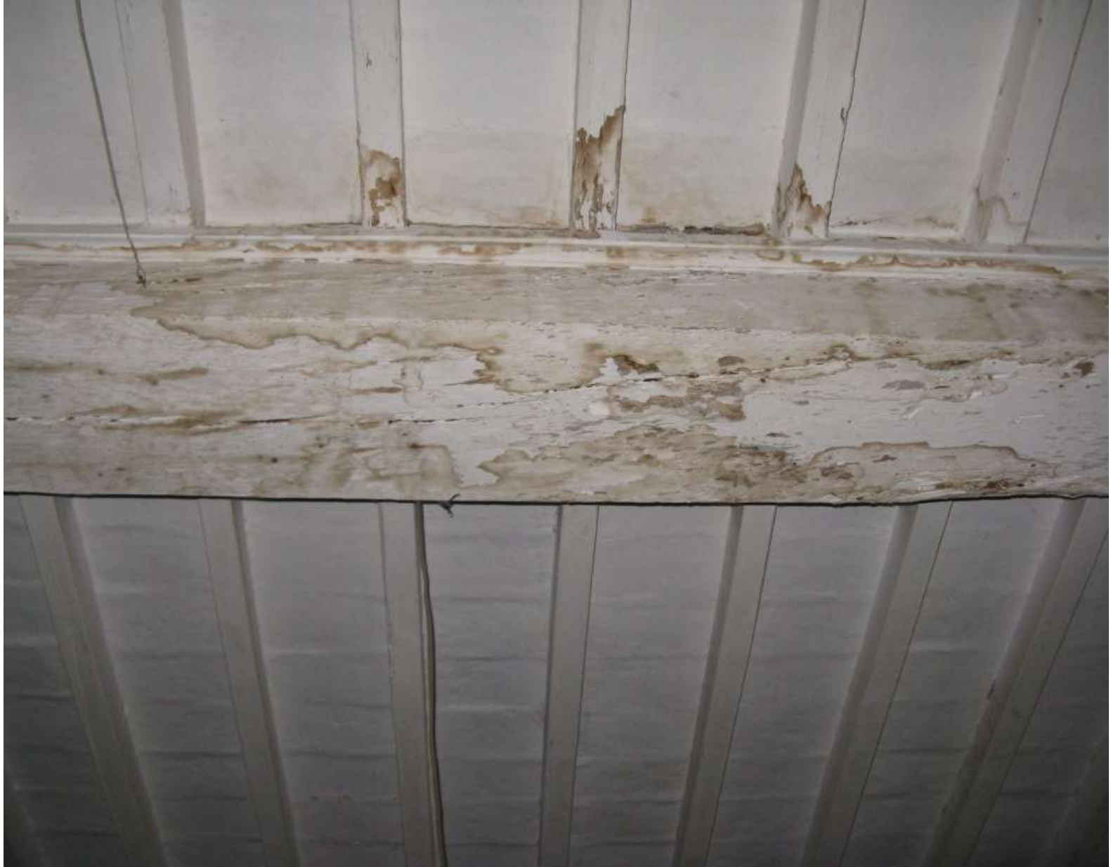
Crack pattern in a beam
